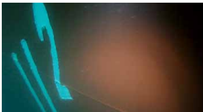
Figure 11 shows the condition of the first full HEMPAGUARD ship applied after 14 months of operation. As can be seen from the figure, the coating was in perfect condition and completely slime free.
